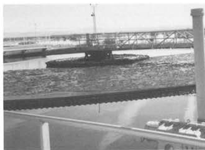
Fred Hervey Water Reclamation Plant
