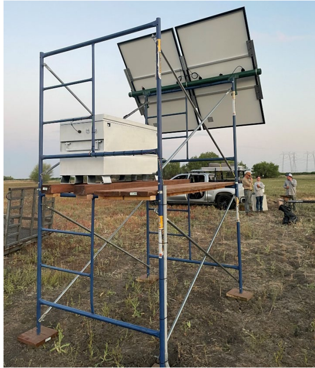
Figure 17. Tower for Solar Power System. The displayed configuration shown has a double stack of scaffolding and twin solar panels.
