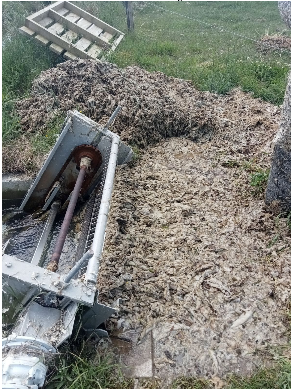
Figure 4 – Image of didymo captured on mechanical pipe intake screen
