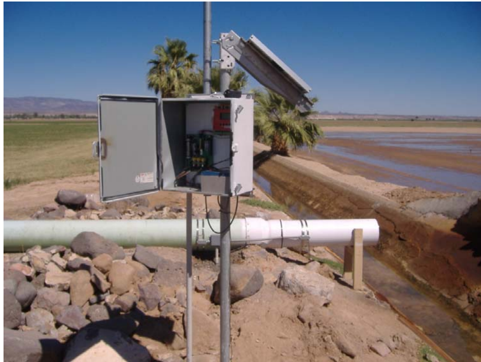
Figure 6. MVIDD pipe fitting venturi meter demonstration site
