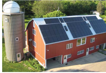
Utilizing existing farm structures for PV
