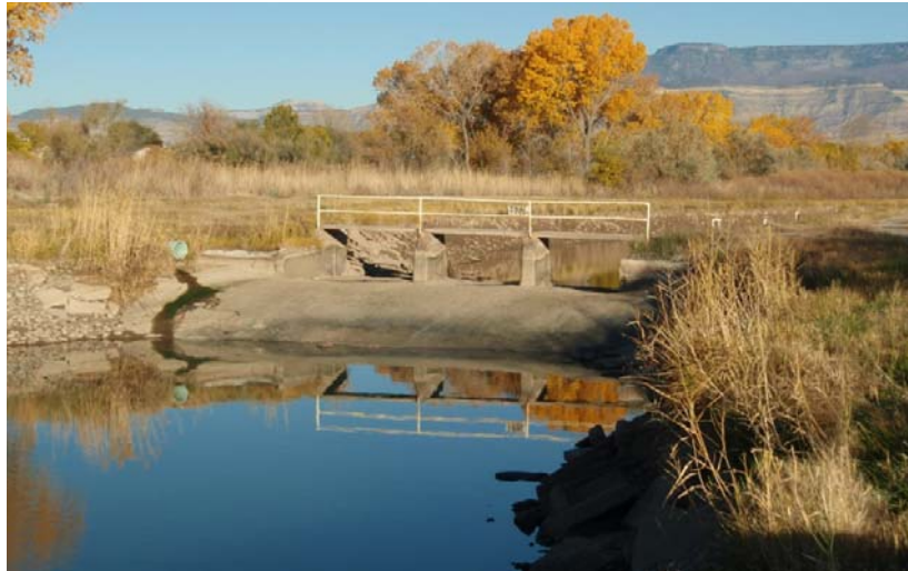
Figure 3. Photograph of Gates Check
