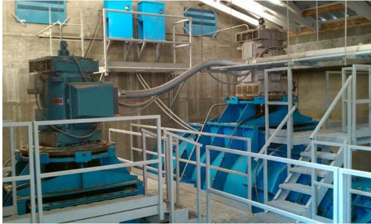
Figure 8. Kings River Siphon Power Plant
