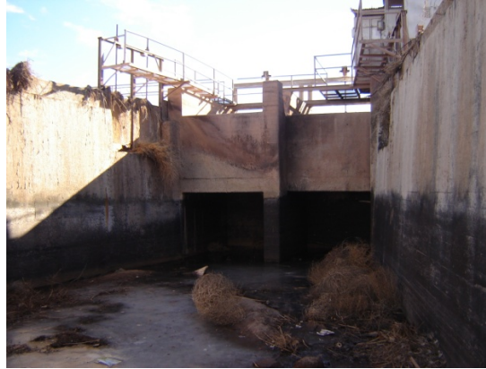
Figure 9. Drop associated with Albuquerque Main Canal Check #1
