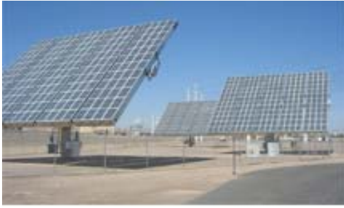
Pole Mounted CPV with work around space
