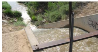
Figure 5. Steep chute at lower Tebo Feeder
