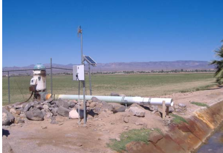
Figure 2. Pipe flow measurement field test site at MVIDD well 23
