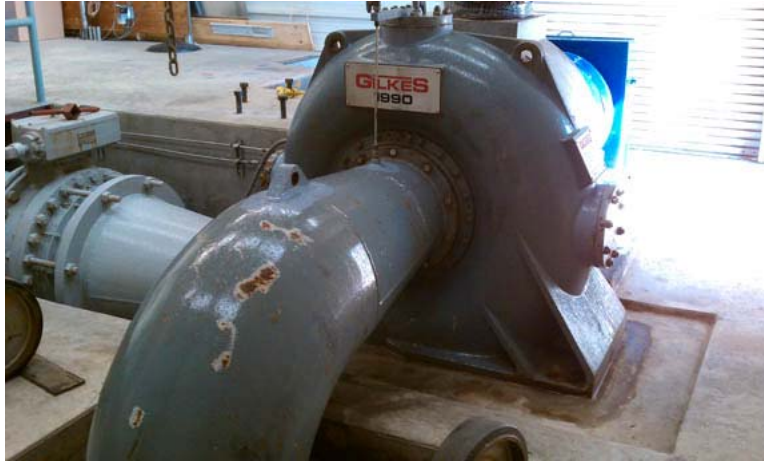
Figure 10. Turbine at Fishwater Powerplant
