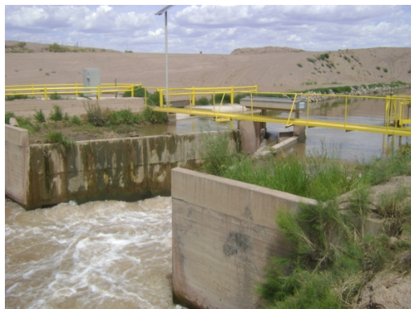
Figure 11. Drop at Polvadera Check
