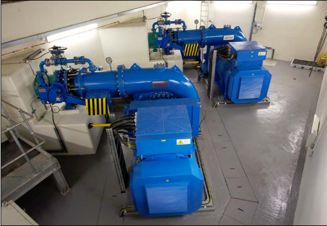
Figure 5. Similar Off-Set Installation by Gilkes
