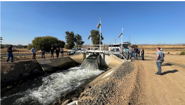
Photo 1: Updated Check Structure at SID
