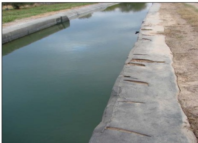
Figure 6. Cuts/tears in a rubber liner
