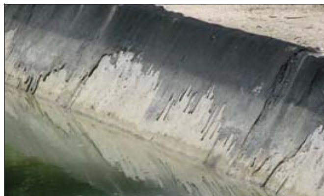
Figure 9. Residue left from a deteriorated polyurethane liner
